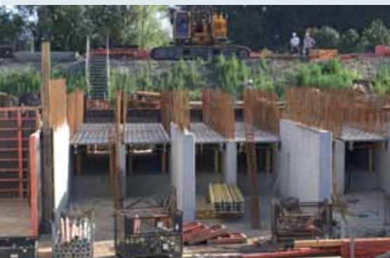
Figure 7.8. Formwork and reinforcement of the intermediate plate of the inlet and outlet
